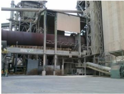
Cement Kiln furnaces in Holcim Philippines
